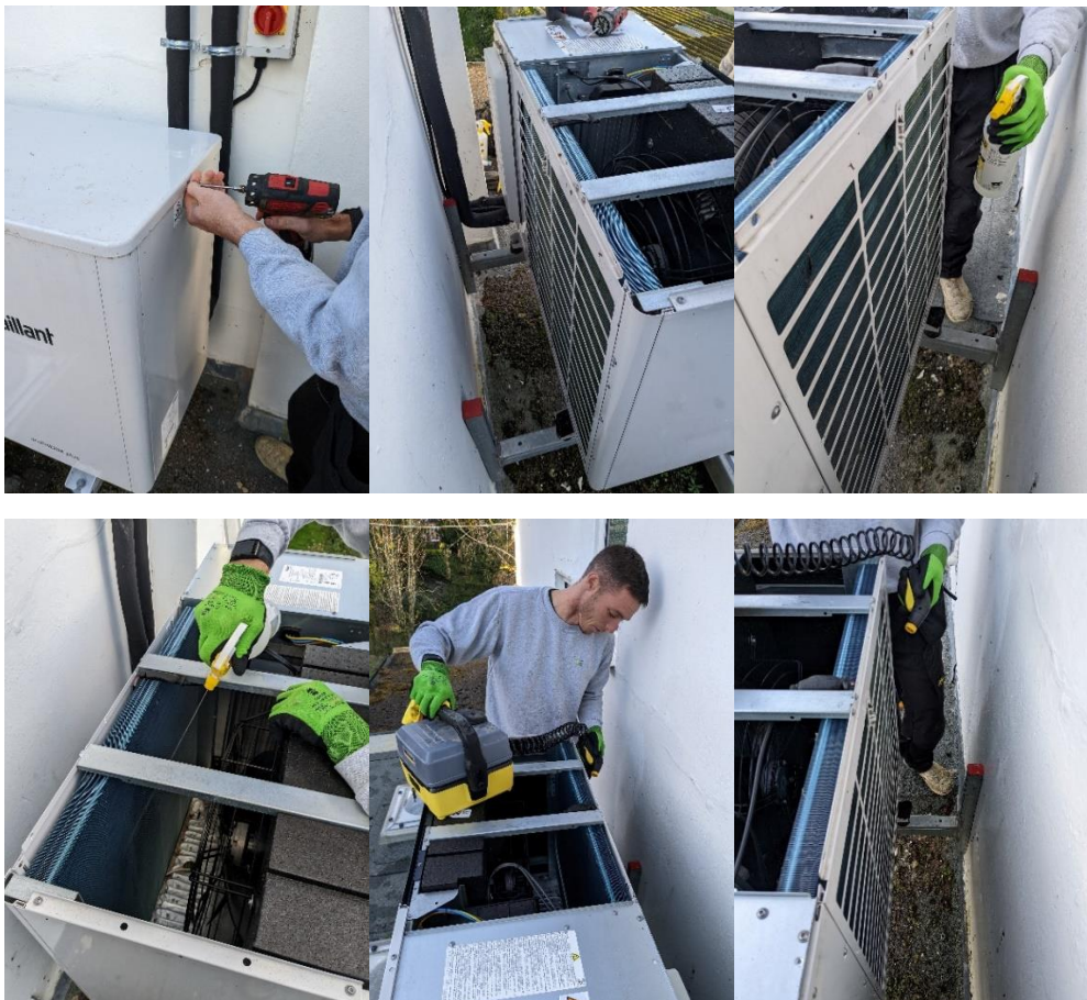
Pic.2 – Example Vaillant aroTHERM Plus unit evaporator clean
