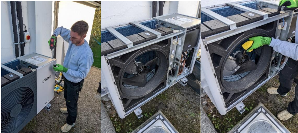
Pic.4 – Cleaning of outdoor unit facia
