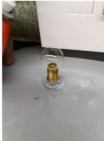
Pic.8 – Failed Schrader valve
