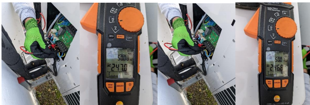
Pic.10 – Electrical checks on ASHP (L-E & L-N)
